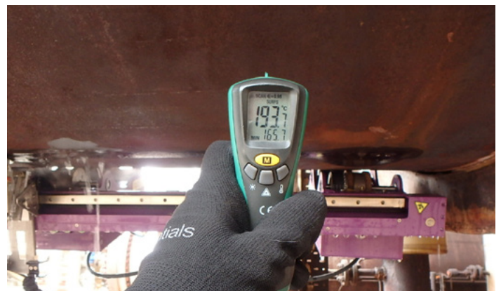
Elevated surface temperature
